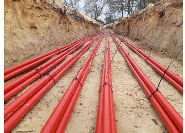
Medium voltage cables
