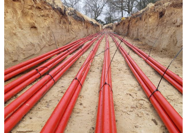
Medium voltage cables
