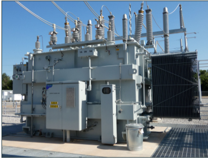
Figure 4: Large power transformer a
